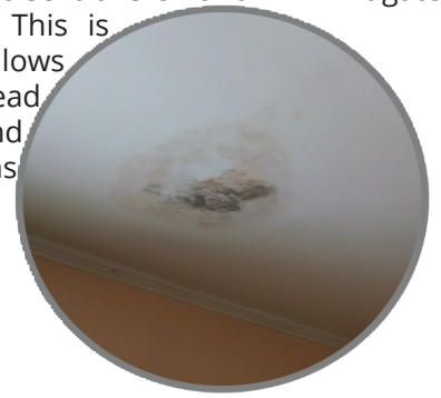
Mould accumulation due to water penetration from building envelope
